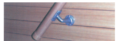
Stairway handrail bracket stop
